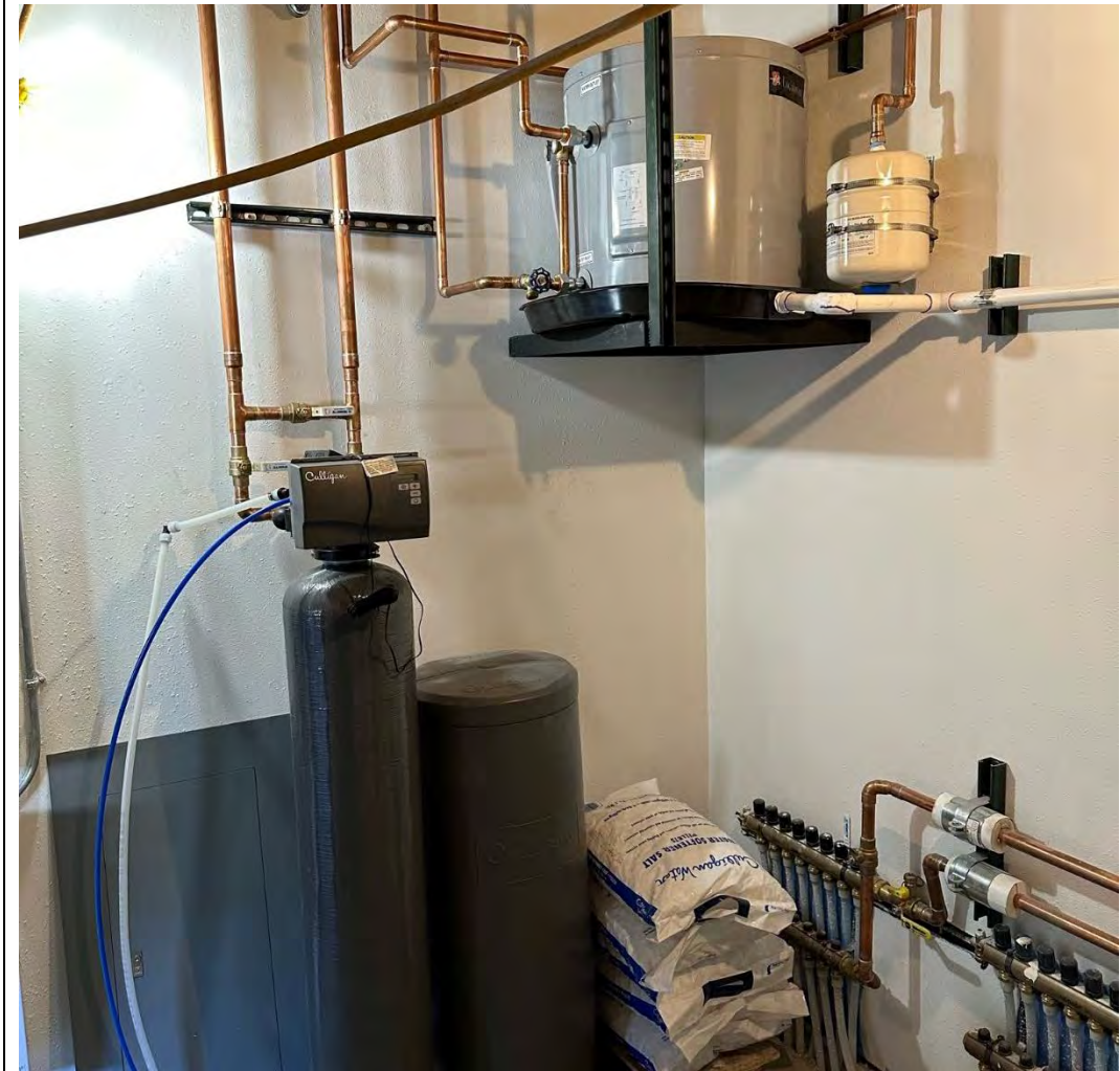
4. Plumbing Equipment for Domestic Water Hooked-Up.
